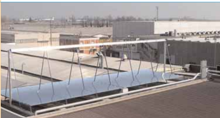
Task 33 Demonstration Project in Bergamo, Italy. The PSE linear Fresnel Process Heat Collector powers two NH 3 /H 2 O absorption chillers.
