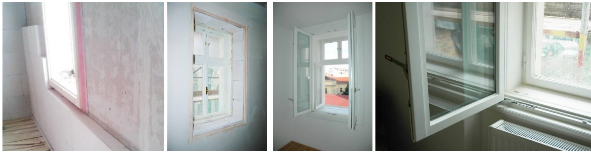
Figure 31: Replacing of inner window layer, © Courtesy of Trimmel Wall Architekten ZT GmbH
