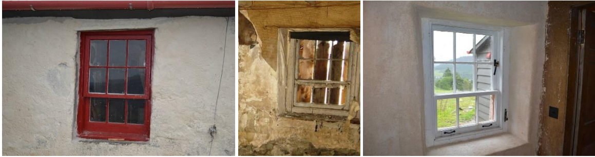
Figure 6: Example taken from ATLAS case Downie's Cottage. Single window before and after repairing, © HES
