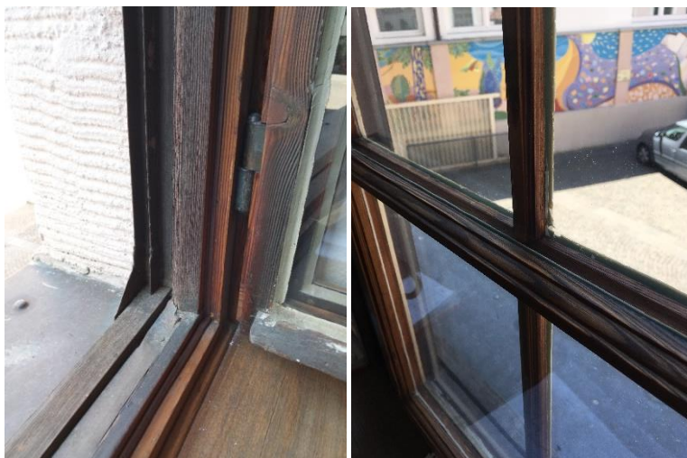
Figure 8: Coupled window with inserted sealing in a groove all around the rabbet
