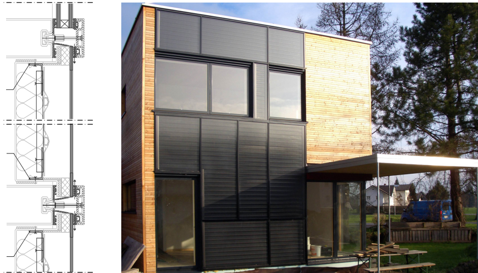
Fig. 3.A.14: Façade integration of glazed flat plate collectors as façade cladding, detail and picture.
