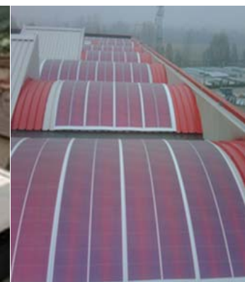
FLX-MO Installation Vigonovo di Fontanafredda (I), © VHF – Technologies
