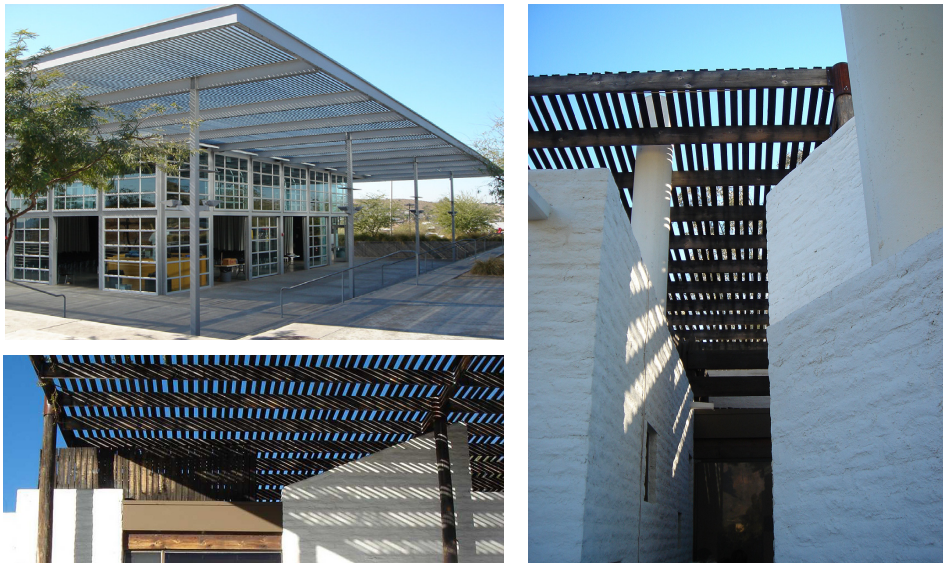
Fig. 3.A.20-a-b-c: Examples of double roofs conceived to reduce building heat (a: double tin roof in Arizona architect n.a; b and c: double roof on a private house in Arizona. Architect Judit Chafee, credits Marja Lundgren).
