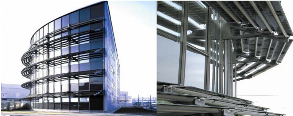
Fig. 3.B.29 SBL Offices Linz, Austria, Helmut Schimek, shading louvres with integrated photovoltaics and suntracking system, © Colt
