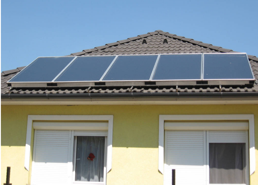
Fig. 3.A.21 Typical standard glazed flat plate collectors installed over the roofing, as purely technical add-on
