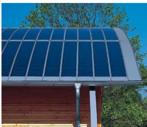
Solar PV Standing Seam System on a curved roof, © RheinZink
