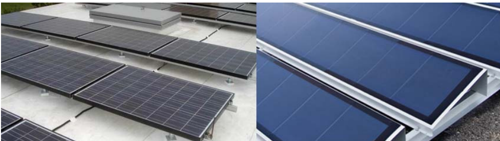
Fig.3.B.19: crystalline modules for flat roof. Left: standard module on rack mounting system, © Prosolar Right: special rack system for flexible laminate on stainless steel substrate, © Unisolar.
