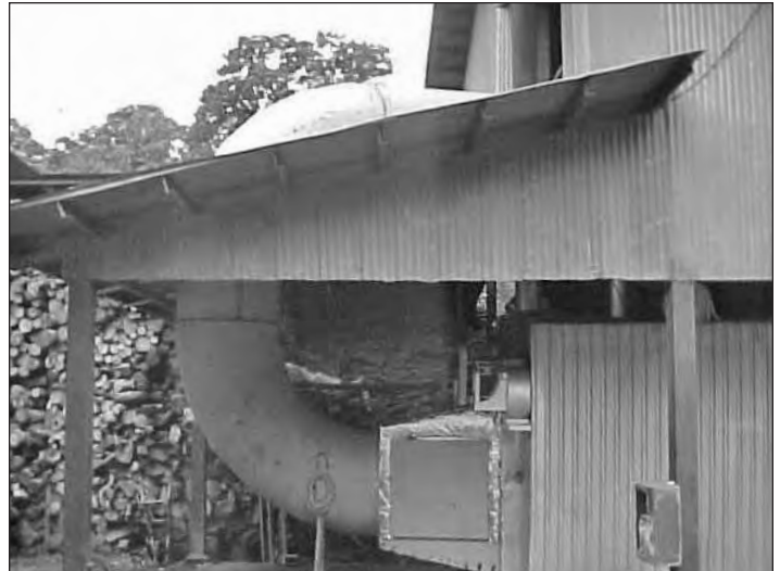
The Coopeldos coffee drying system in Costa Rica has now operated successfully through a drying season. Shown above is the duct from the solar panel entering the furnace.
