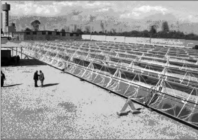
Figure 10. The EI NASR Pharmaceutical Chemicals facility in Egypt has an installed capacity of 1,33 MWth
