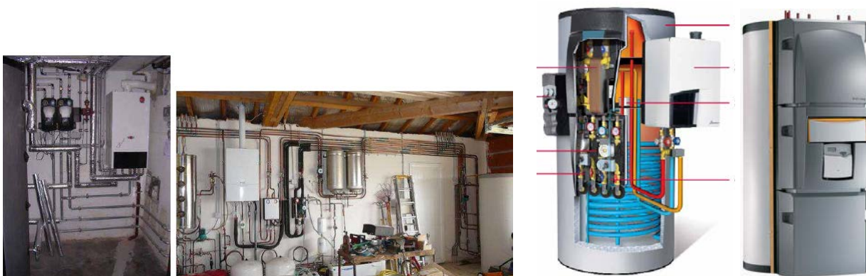
Fig 2. Examples of often existing bad hydraulic installations (left) and examples for compact solutions with minimized pipe length within the system (right) [4]
