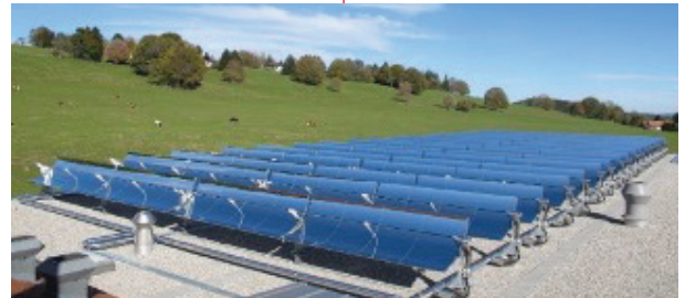
Emmi Dairy Saignelégier in Switzerland uses parabolic trough collectors to generate steam for different dairy processes. (Source: NEP Solar AG / SHIP database, http://ship-plants.info/ )
