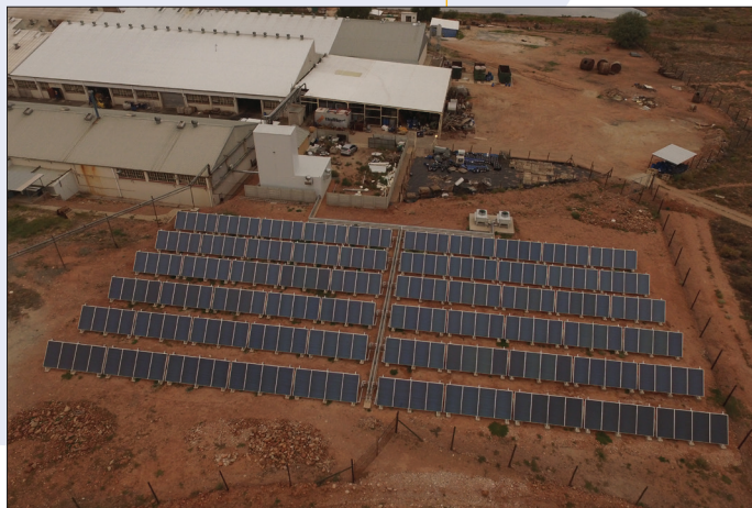
▲ Figure 2. Ground mounted system at the Klein Karoo tannery.
