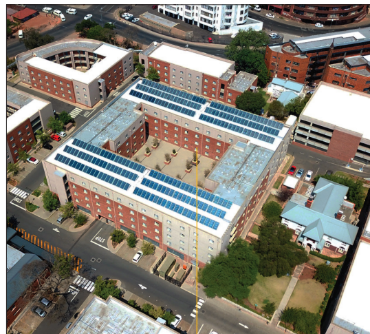
▲ Figure 1. District heating system on the Wits Junction residence building combines solar thermal, co-generation and gas technologies
