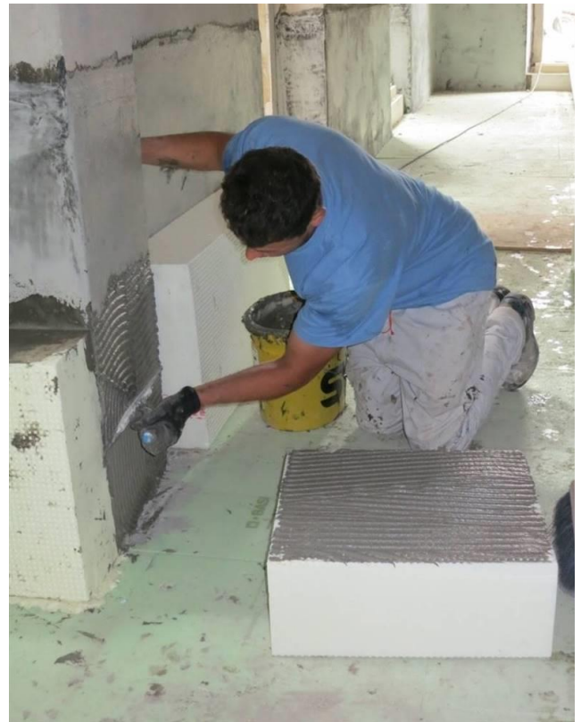
Interior insulation with perlite was installed where possible. Aerogel insulation was used elsewhere.
