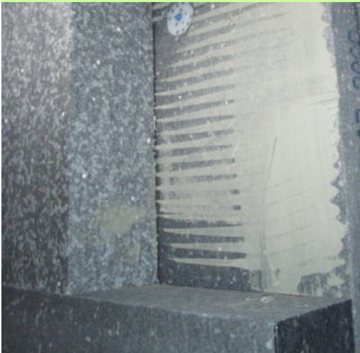
Wall exterior insulation
