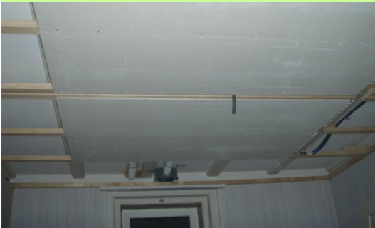
Radiant suspended ceiling
