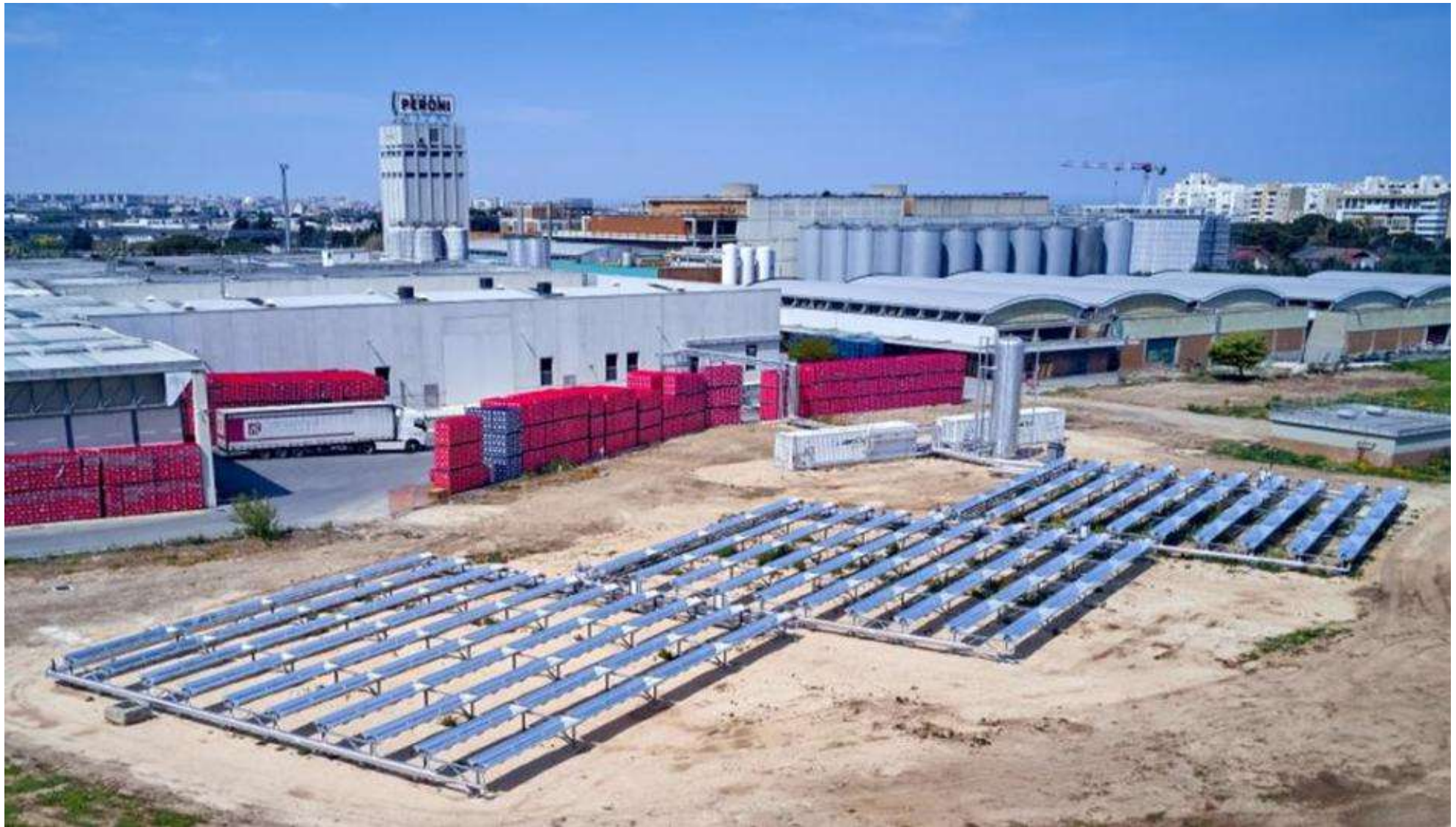
660 m 2 parabolic trough collectors for the Brewery Birra Peroni in Bari, Italy
