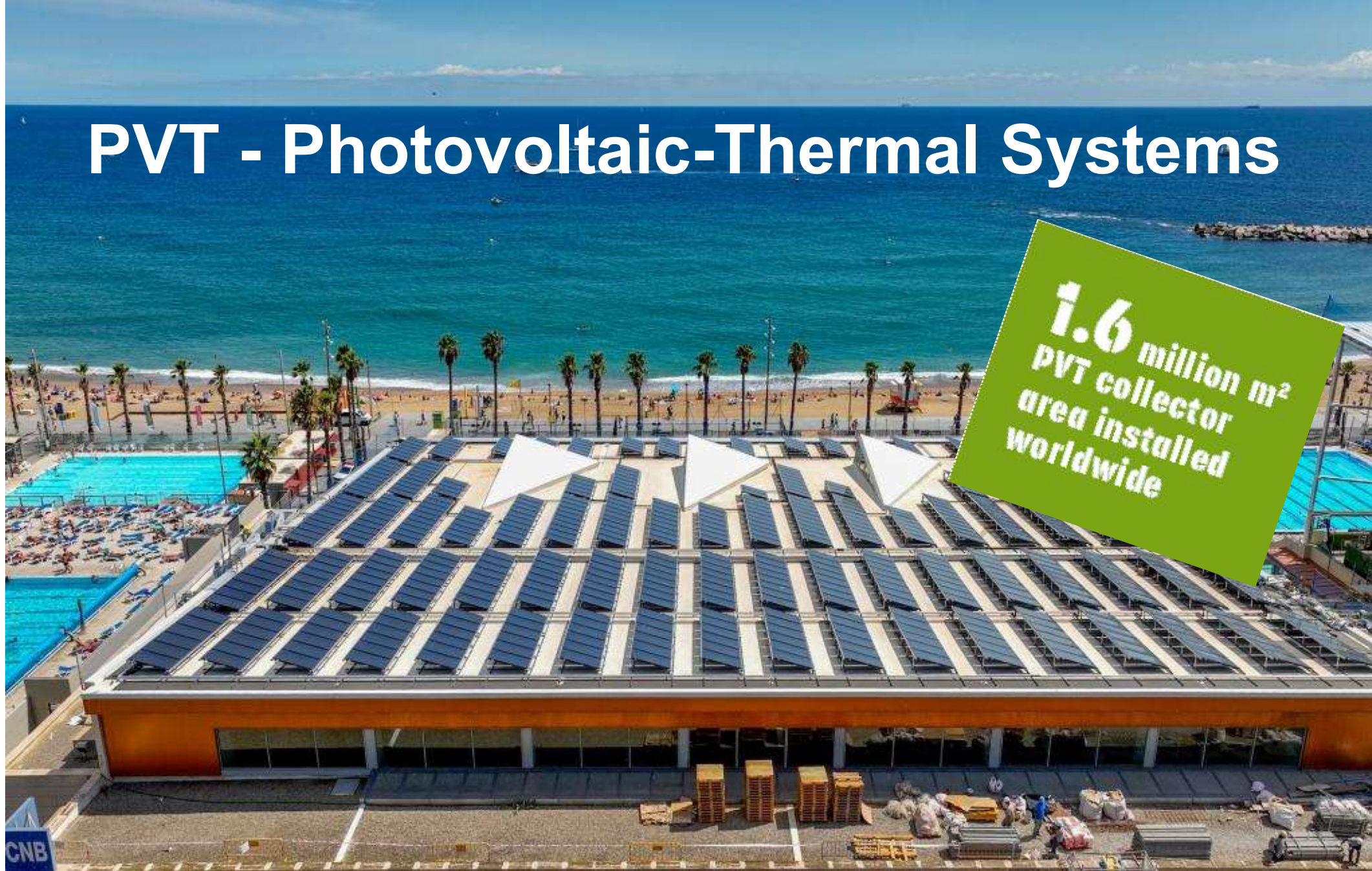
Domestic hot water and swimming pool system with 2,082 m 2 PVT in Barcelona, Spain Photo: Abora Solar, Spain
