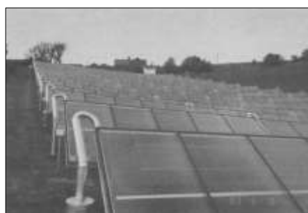
First solar district heating plan in Saltum, Denmark, installed by Saltum Varmevaerk.
