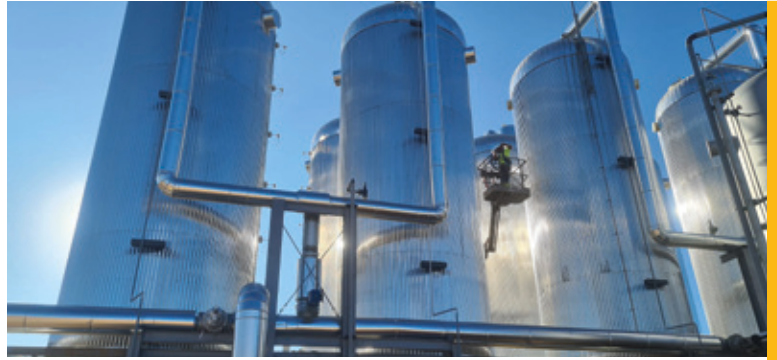
Heat storages for the Heineken brewery in Seville, Spain Photo: Engie, Spain
