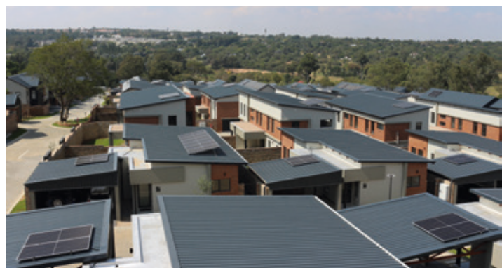
PV2Heat systems installed in South Africa Photo: Bongani Xakaza, SANEDI, South Africa
