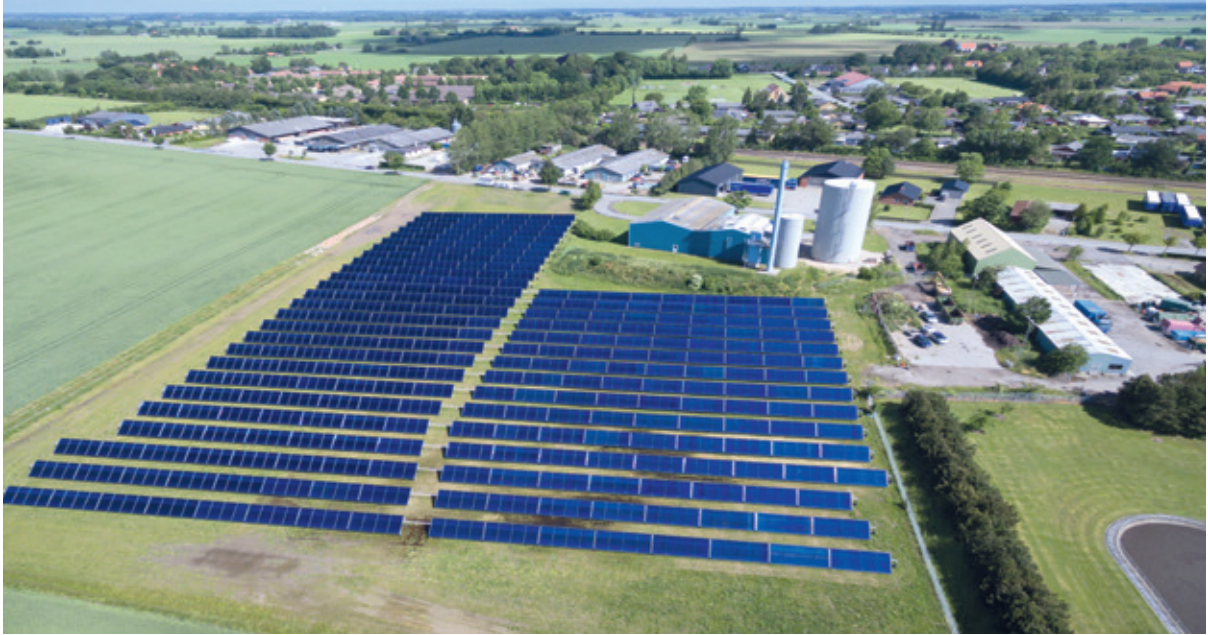
Solar district heating plant in Søllested, Denmark, consists of 4,700 m 2 double glazed flat plate collectors
