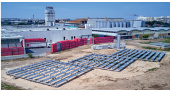
660 m 2 parabolic trough collectors for the Brewery Birra Peroni in Bari, Italy
