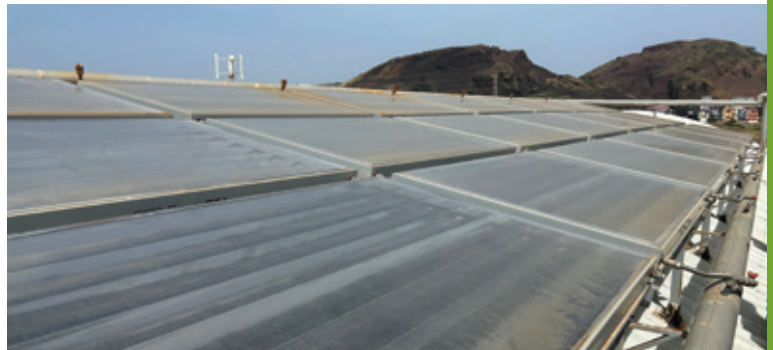
Heat from 294 m 2 of flat plate CPC (Compound Parabolic Collector) solar collectors drive a 70 kW water/LiBr absorption chiller for air-conditioning at the CERMI center in Praia, Cape Verde, since 2013 Photo: JER
