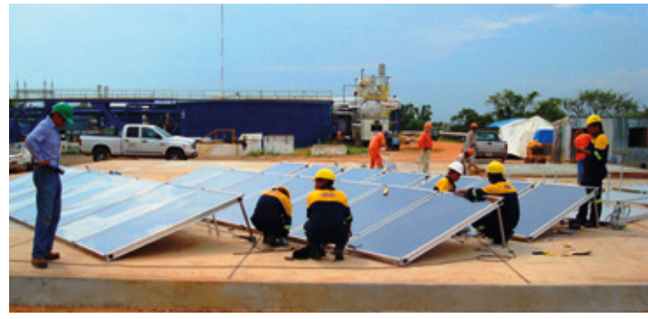
Flat plate collector system in Mexico Photo: Mexichem / Solar Payback
