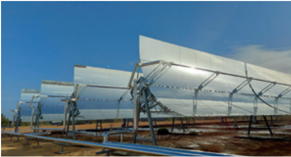
A section of Europe's largest solar industrial heat plant, with a capacity of 30 MW th , was installed by Engie in cooperation with Azteq-Solarlite Spain at the Heineken brewery in Sevilla, Spain
