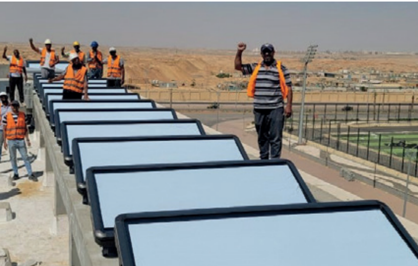
Installation of Sunpad systems in Cairo, Egypt Photo: GREENoneTEC Solarindustrie GmbH, Austria
