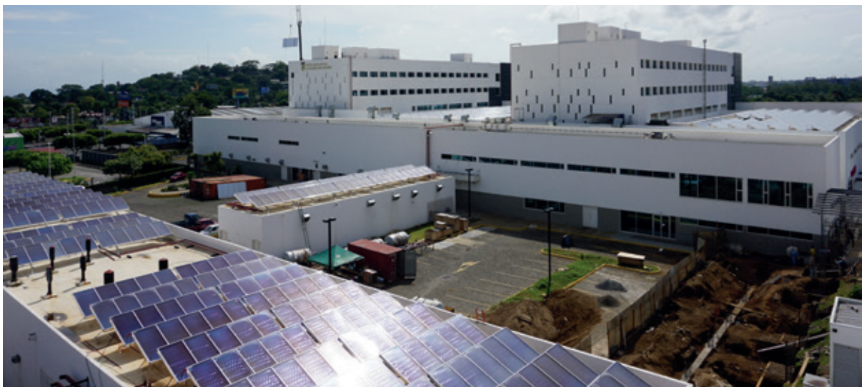
1 MW Solar cooling system at the Hospital Militar Escuela in Managua, Nicaragua
