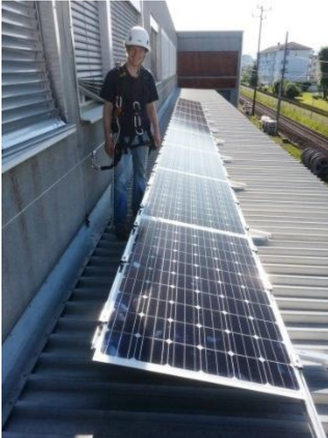
PV modules (Meyer Burger) – south oriented
