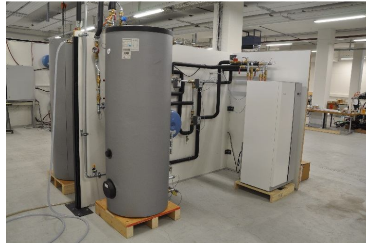
Cooling machine (HP; ait / Nibe) & storage tanks.
