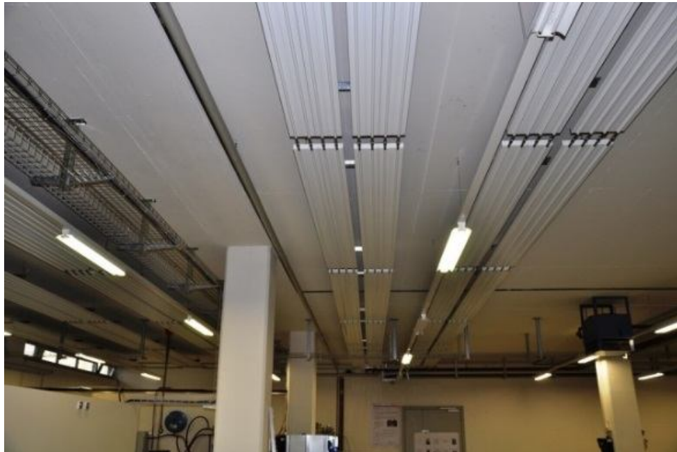
Cold ceilings (Zehnder) installed in the Laboratory (52.5m 2 ).
